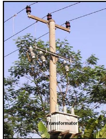
Gambar 5.9 Transformator Distribusi Tipe Tiang
